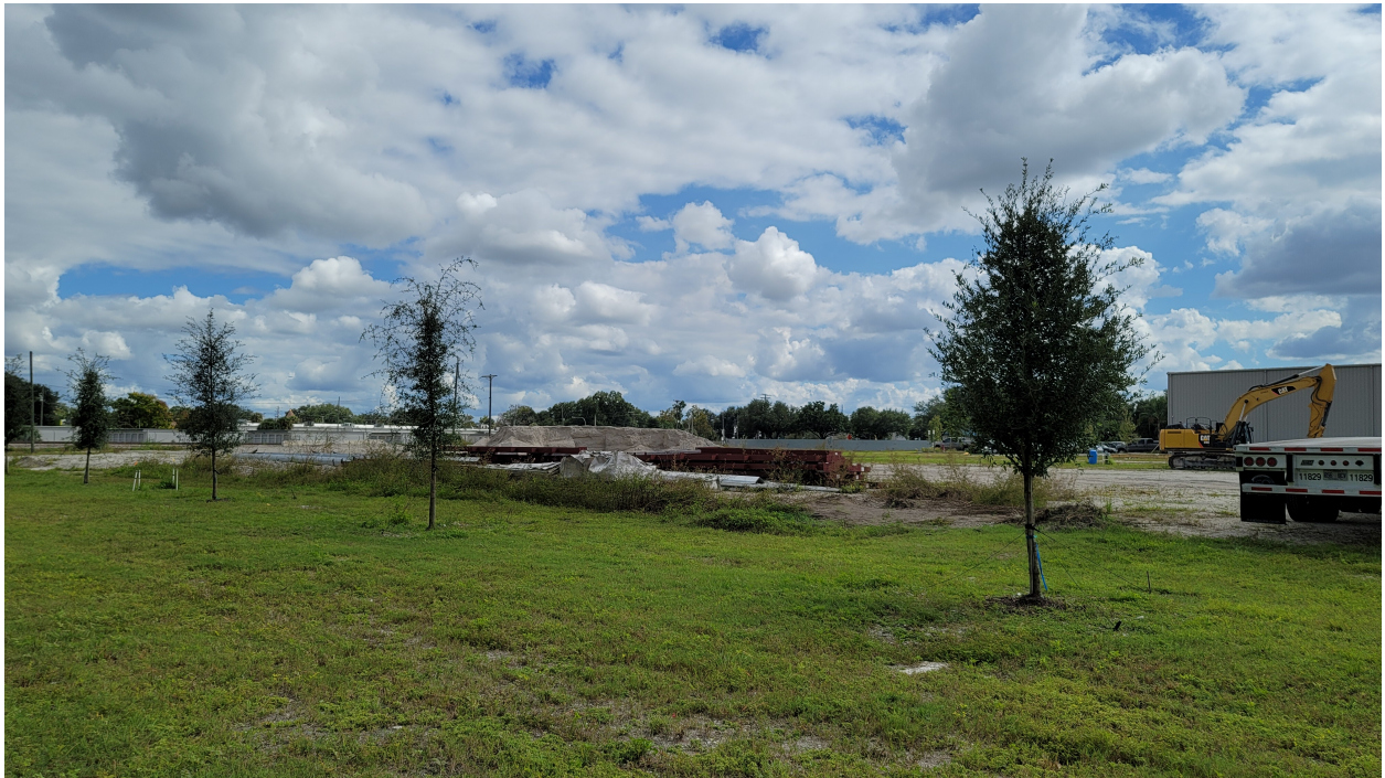
Photo 5: Looking southeast towards existing construction materials which have been stored on-site. Grass overgrowth is to be removed by the Owner.
