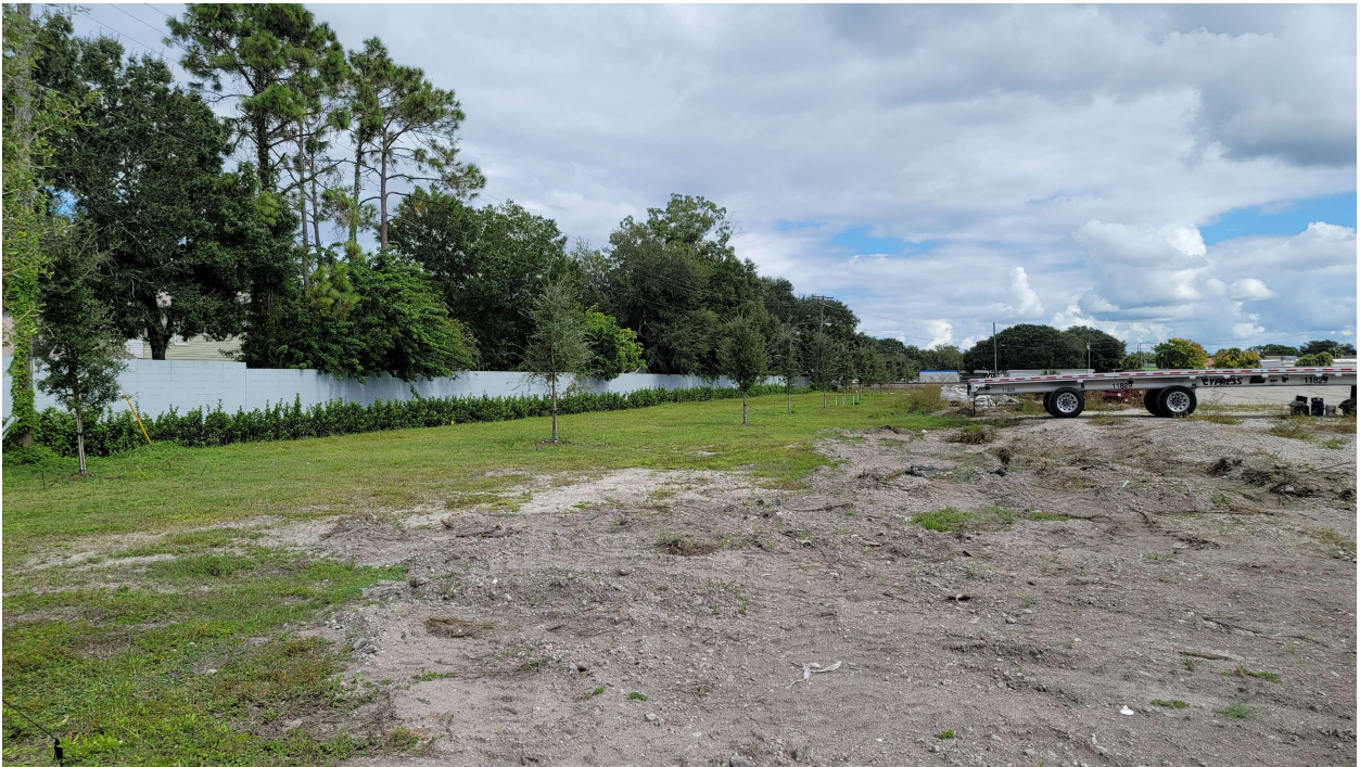
Photo 3: Looking east along the northern landscape buffer area where debris has been cleared.
